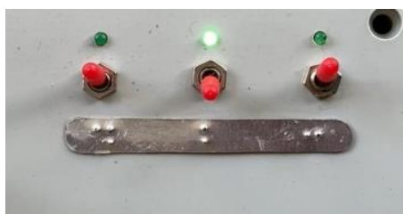
Figure 15. Switches to change the operating mode.
